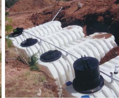
Belowground Water Cisterns
