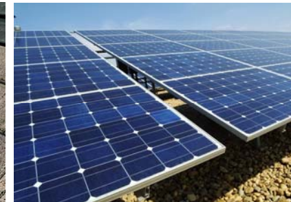
Solar Energy Generation
