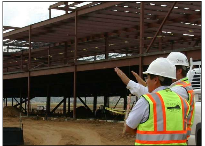
Town Manager Andre Cordero touring the new IHS Hospital with a Flintco, INC. representative.
