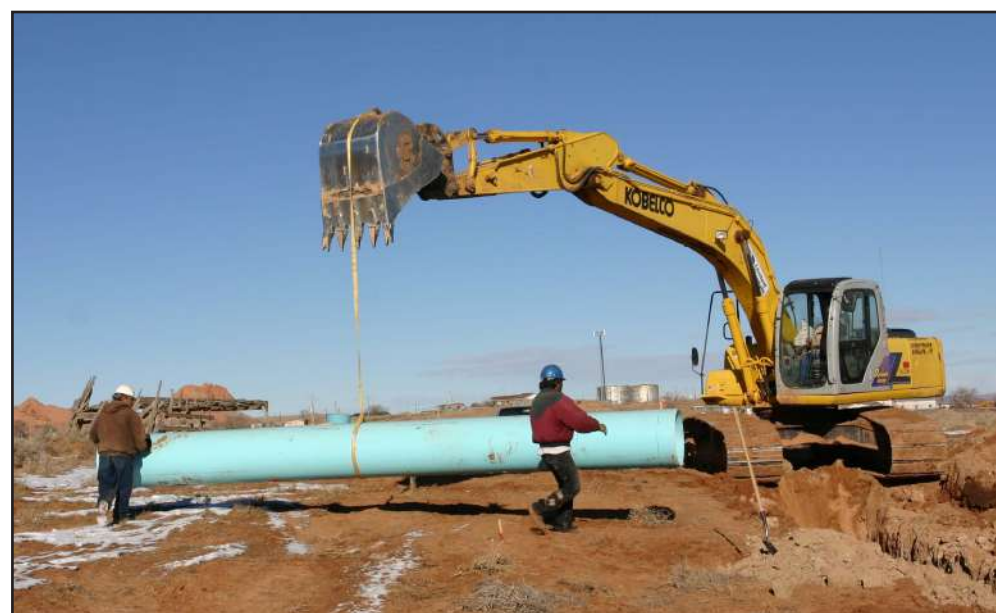
December 21, 2007, waterlines were being put in the ground in the Kayenta area for the Farm Board project.
