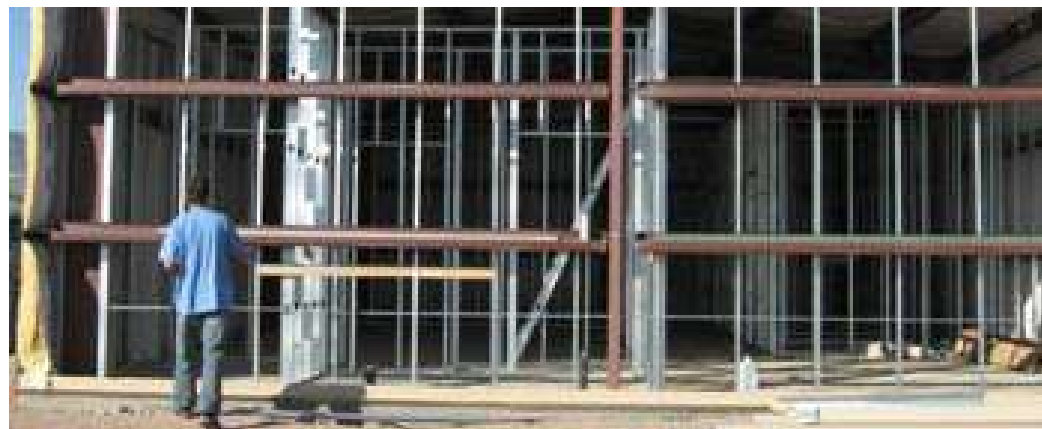
Pictured: The new Kayenta Animal Shelter during its construction phase, located just off Highway 163 in Kayenta.
