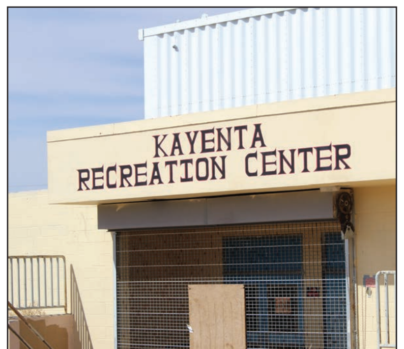
KAYENTA, ARIZ. - Kayenta Recreation Center fenced in to maintain safety is scheduled for demolition. There are plans to build a new facility.
