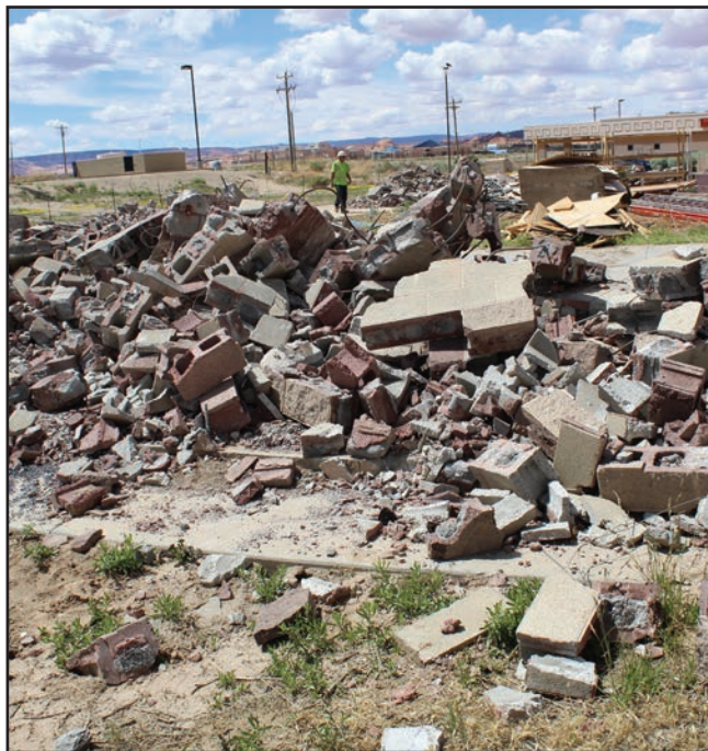
KAYENTA, ARIZ. Construction debris from the building are piled and hauled away to Transfer Station for recycle.
