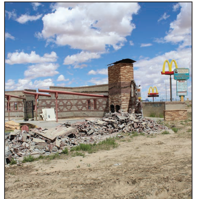
KAYENTA, ARIZ. - The interior of the building can be seen as the demolition begins with tearing down east side of the structure.
