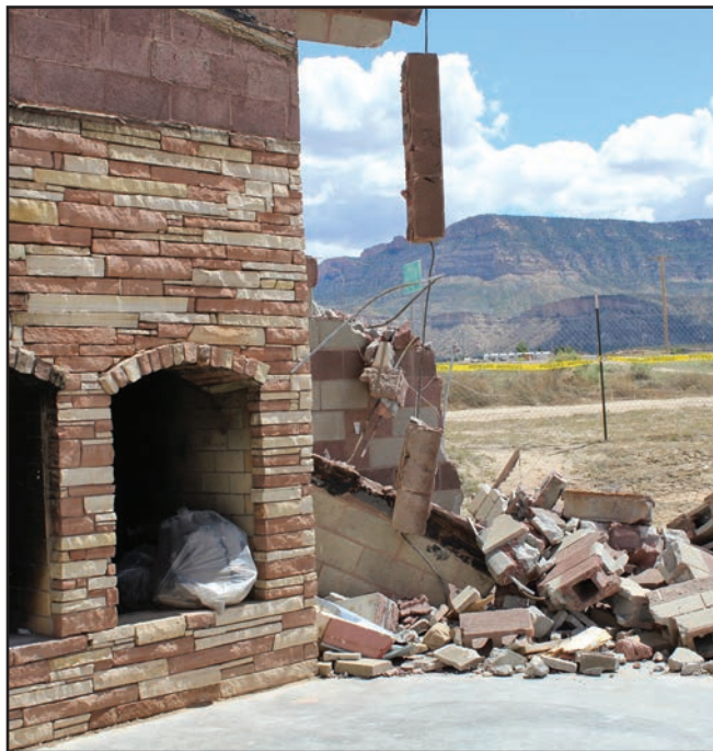
KAYENTA, ARIZ. - Fireplace set to be demolished. Black Mesa view in the background by US HWY 160.
