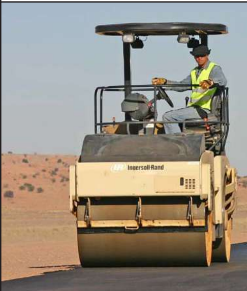
The reconstruction of the Kayenta Airport was a major milestone in the Townships Capital Improvement Plan.
