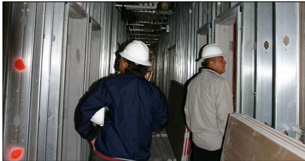
Kayenta Township employees Gabriel Yazzie and Milton Crank look over the construction process inside the new KCS dormitory.
