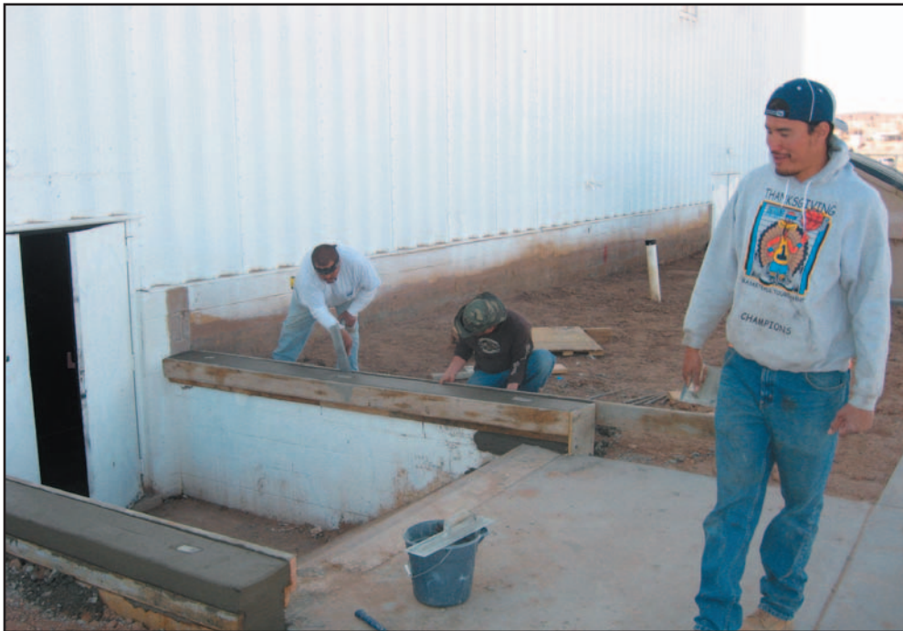
Kayenta Township Construction Crew fixing the rear entrance of the Recreation Center.
