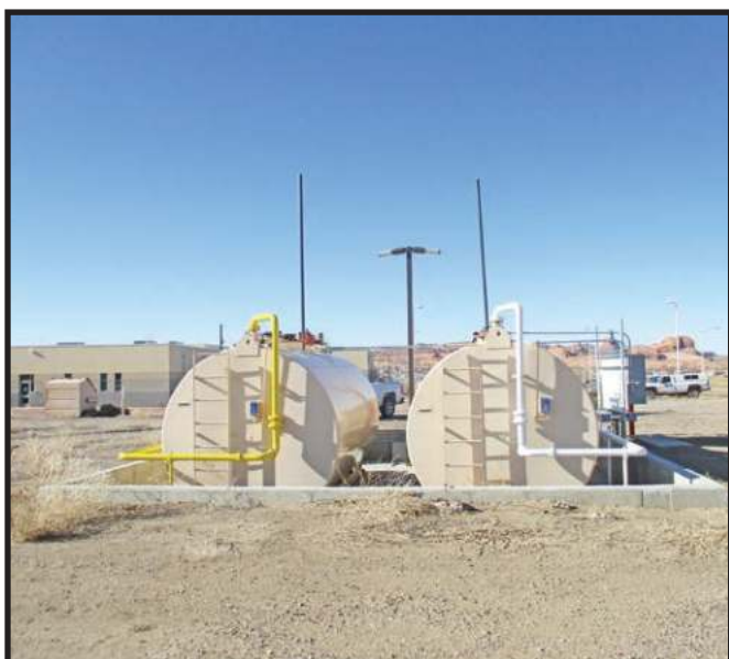
Kayenta, Ariz. - New Fuel tanks at Correctional Facility and Kayenta Police Department Support Building. (Photo Courtesy of Mark Joseph, KTC.)
