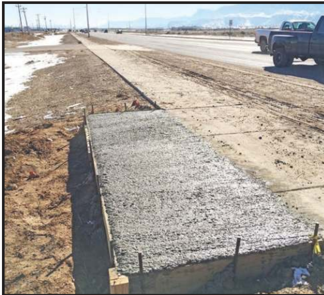
Kayenta, Ariz. - Newly poured concrete for bench placements in and around the Kayenta Township. (Photo Chris Burnside, KTC.)
