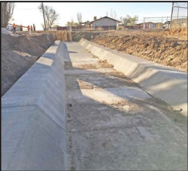
Kayenta, Ariz. - New canal system being built at KUSD. (Photo Chris Burnside, KTC.)
