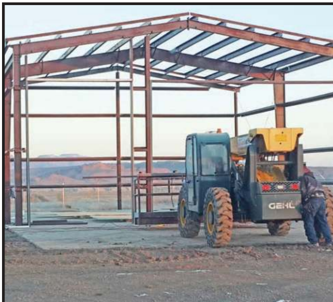
Kayenta, Ariz. - Newly framed 'Snow Removal Equipment' building near Kayenta Airport being constructed. (Photo Courtesy of Tyler Glasses, KTC.)
