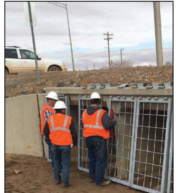
Kayenta, Ariz. Gates were installed near the intersection of US HWY 160 and US HWY 163.
