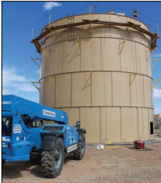
Kayenta, Ariz. A water tank was recently installed a 175,000 gallons insulated fire suppressant tank at the Navajo Nation Police Department
