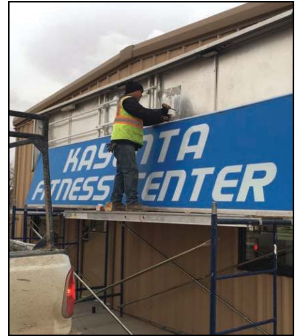
Kayenta, Ariz. Kayenta Fitness Center will soon get a new lights, the lights are being replaced by Kayenta Township employee.
