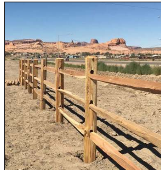
Kayenta, Ariz. A new Cedar Fence was constructed in and around the Division of Public Safety facilities, the fence is part of Kayenta Township Beautification Project. The project is ongoing. You can see the fence near US Highway 163.
