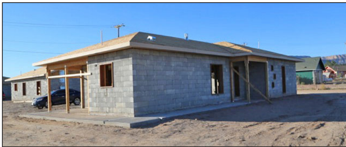
Kayenta, Ariz. New homes under construction, part of a newly 40 homes being developed by Navajo Housing Authority. (photo courtesy of Christian Bigwater, NHA).
