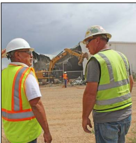
Kayenta, Ariz. Tyler Glasses, Project Coordinator and contractor observe during the demolition of the old Kayenta Recreation Building. The demolition project is complete and area is safe to the general public.
