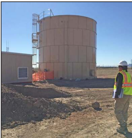
Kayenta, Ariz. a One Hundred Seventy Five Thousand gallon water tank was constructed in the Kayenta Department of Public Safety facilities near the Navajo Corrections and the new Police Department. Mark Joseph, Building Inspector following through with project.
