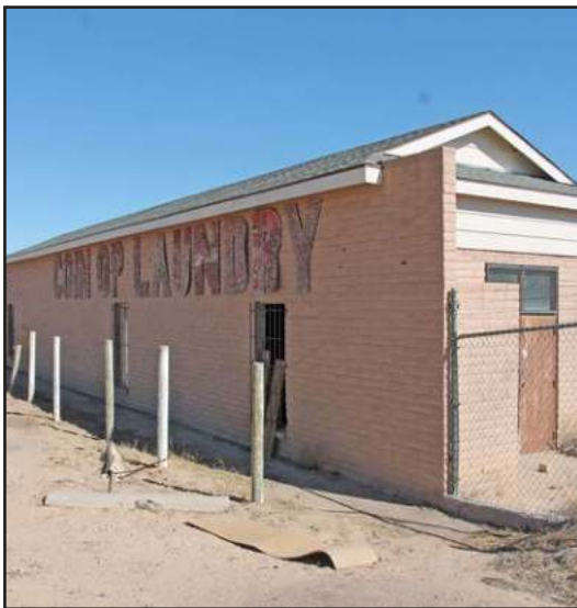
Kayenta, Ariz. The old Coin-Op Laundromat located near the Kayenta Trialer Park is scheduled to be demolished in the month of November 2016.
