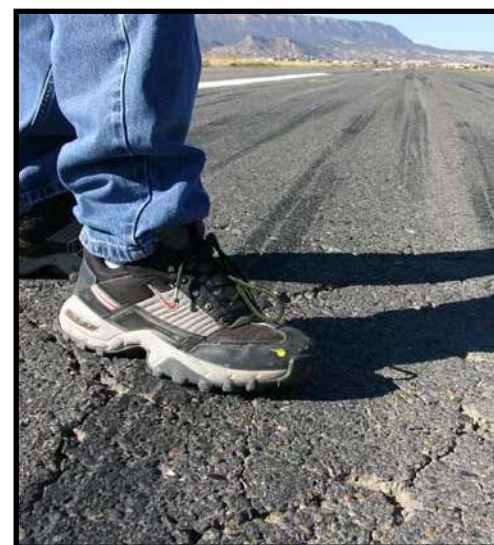
Cracks such as these pictured, litter the existing Kayenta runway.
