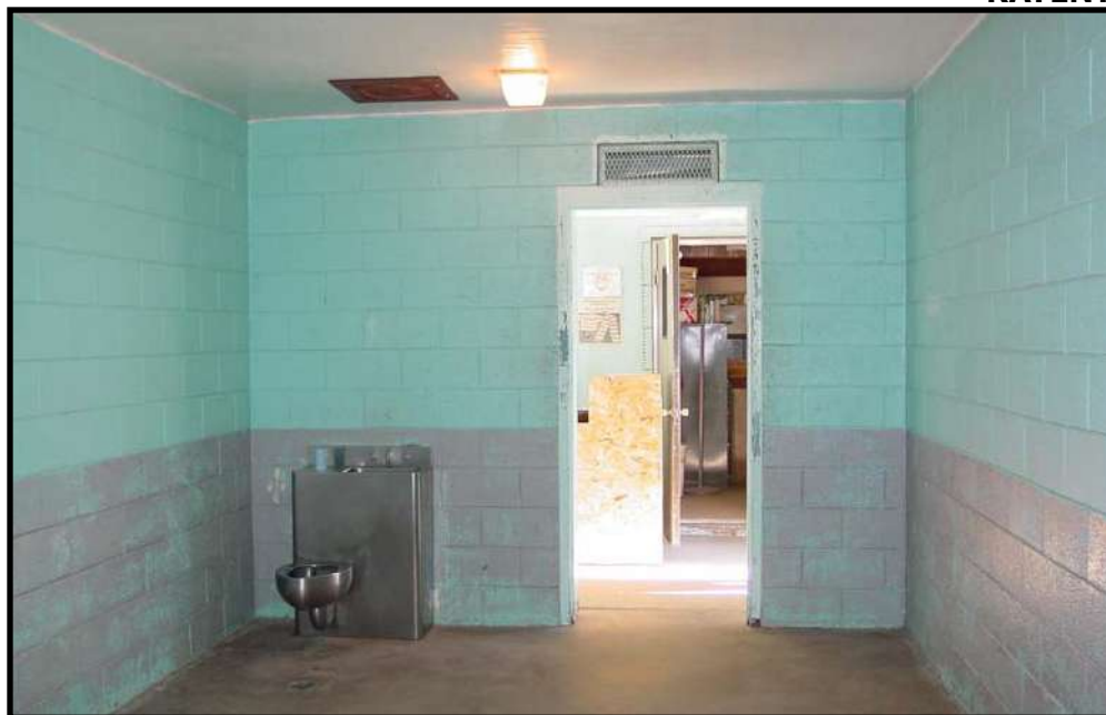
Current jail facilities in Kayenta failed safety standards and posed many violations in fire safety, building structure, and hygiene.
